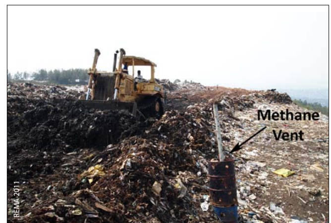
A bulldozer compacting trash at Nyanza near a vent installed to release methane
