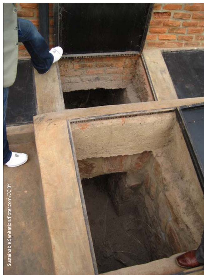
A compost chamber at a school in rural Kigali
