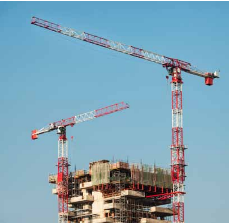
The building sector will be a key area of opportunity in the EU's ambitious climate and energy package. © George Clerk/iStock
