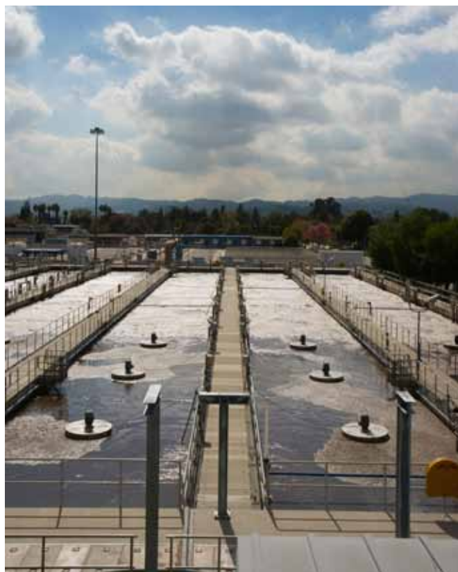
Waste treatment plant, Los Angeles, United States. © John Crall/iStock
