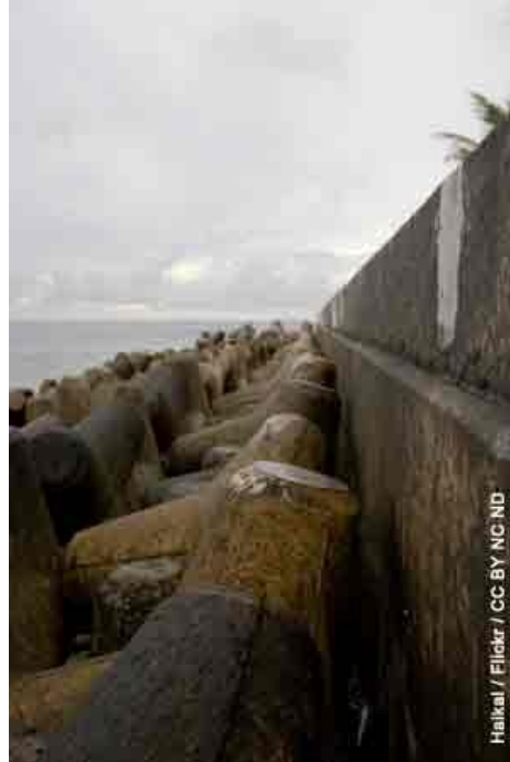
Figure 5: Completed in 1990 at a cost of US$ 70 million, a tetrapod wall was constructed to prevent coastal erosion along the edges of the Male in the Maldives.
